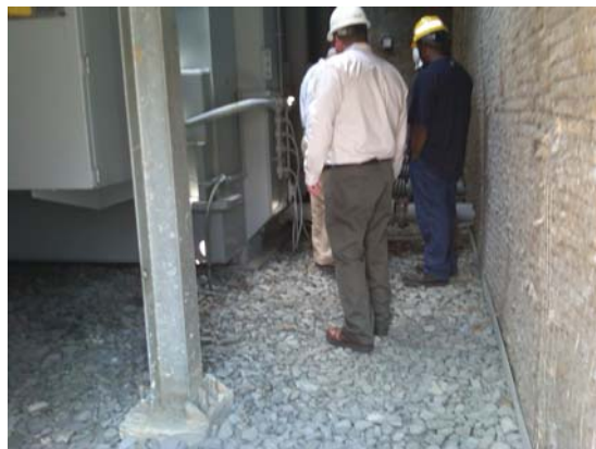
Pepco engineers and environmental cleanup consultants inspecting transformer containment area at the company's Potomac River Substation.
